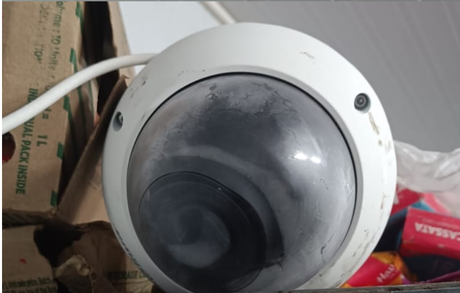
Figure 1-7 Moisture on the surface
