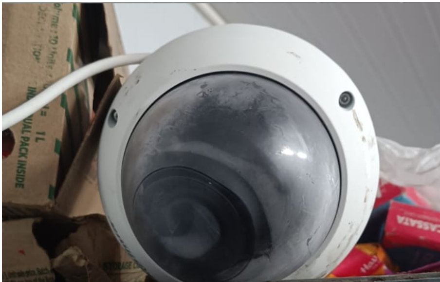
Figure 1-2 Moisture on the surface
